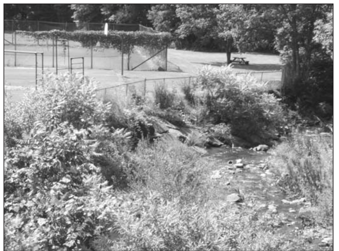
Birch Creek's bank is slip-sliding away in the vicinity of the Pine Hill community playground. A grant to the Town of Shandaken from the CWC's Stream Corridor Protection Program will armor and reseed the bank to prevent further encroachment on the park.
